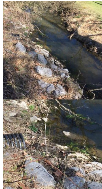
Figure 4b. Site 3 Corrugated Drainage Pipe
