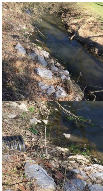
Figure 4b. Site 3 Corrugated Drainage Pipe
